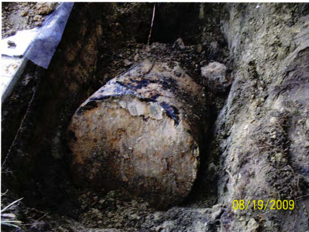
Picture 2: UST 1190Bobwhite.
